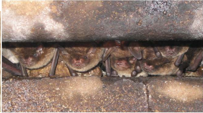
Photo 2: Visible bats within an expansion joint
