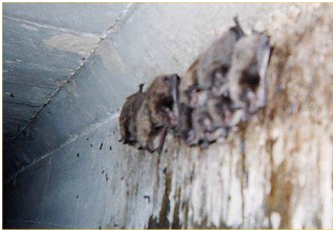
Photo 1: Bats hanging from cracks along Support beams
