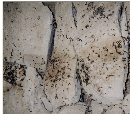
Photo 6: Bat Guano on Riprap
