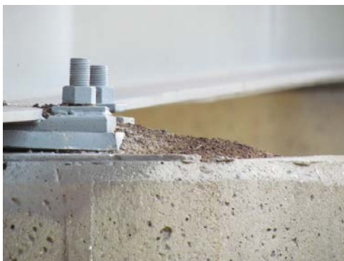
Photo 5: Guano deposit on pier, obscuring structural features.
